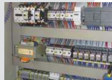
Switching cabinet / SPS control
